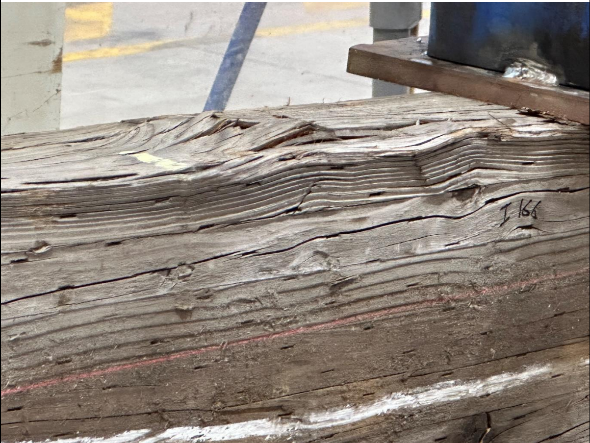
Plastic deformation in Andrew's repaired beam
